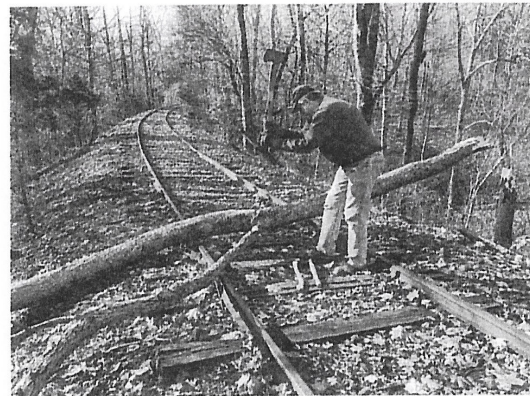
Dave Williamson clearing one of the downed trees near High Trestle Fill. November 14, 2020.
